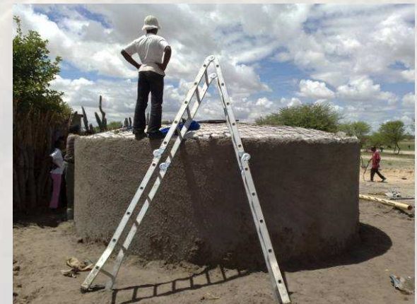
roof catchment with ferrocement tank
