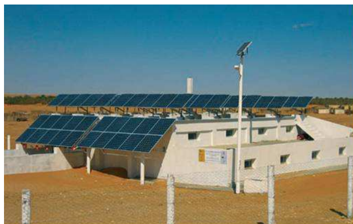
Figure 2: 10.5 kWp solar electricity-operated reverse osmosis of brackish water in Tunisia with a fresh water output of 15 m 3 /day [WISIONS, 2008]
