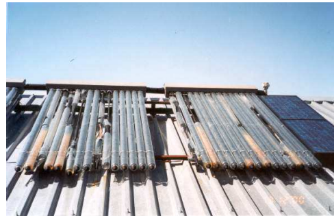
Figure 10: Broken vacuum tubes of TAS solar panel after a hail storm [Stöck, 2004]
