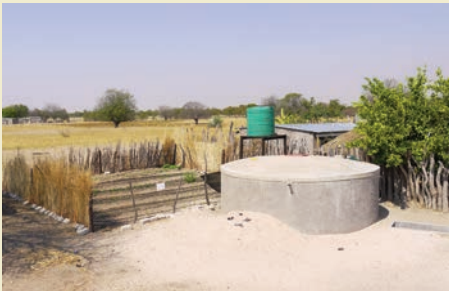
The ferrocement tank constructed within the project with the little garden attached to it for the sustainable use of the rainwater harvested
