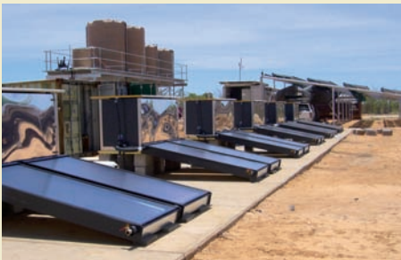
Desalination plants in Amarika (top) and Akutsima (bottom)
