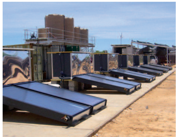
CuveWaters desalination plant in Akutsima, Namibia
